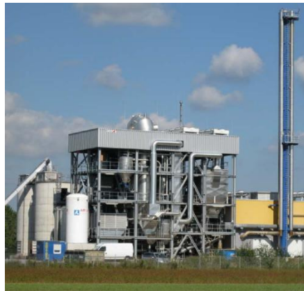
33 GJ CHP ORC plant
